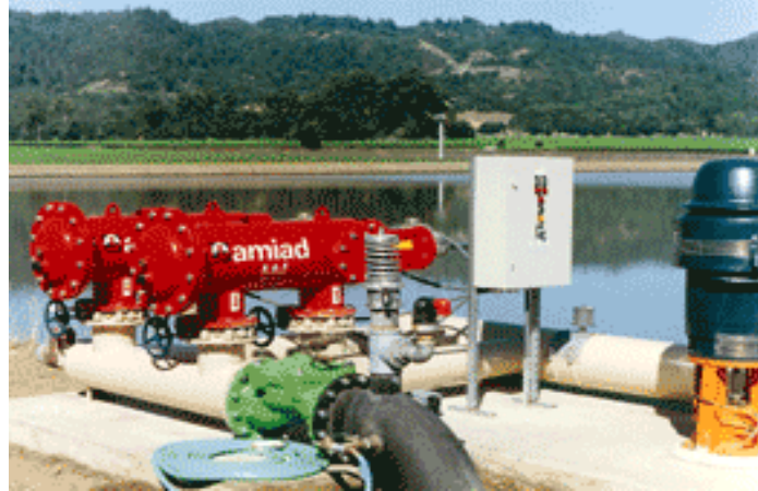
FIGURE 3 130-MICRON FILTERS AT MONDAVI VINEYARDS DRIP SYSTEM, OAKVILLE (COURTESY AMIAD USA)
