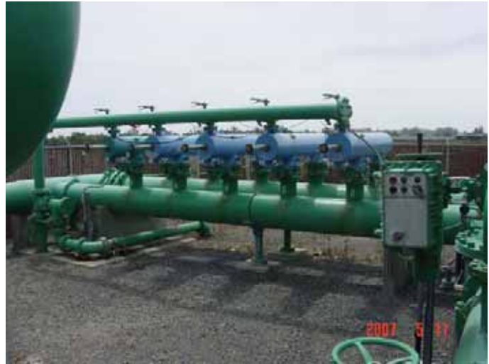
FIGURE 1 ROHNERT PART PUMP STATION FILTERS
