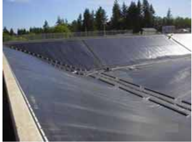
FIGURE 4 FLOATING RESERVOIR COVER (COURTESY MPC CONTAINMENT)
