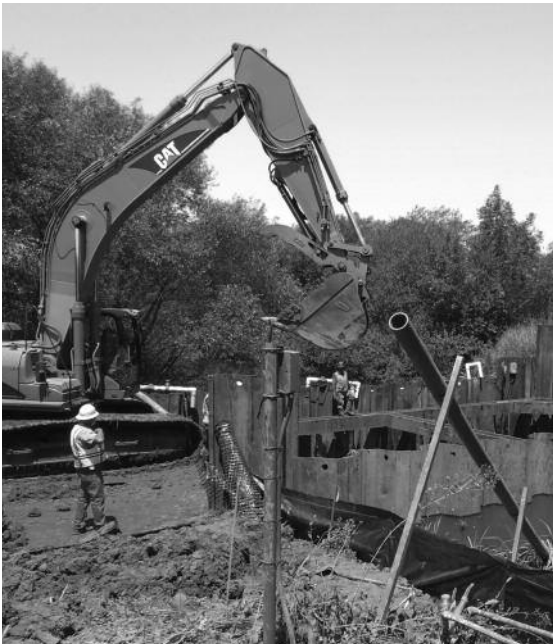
The location of the Discharge Compliance diffuser project presents many construction challenges.
