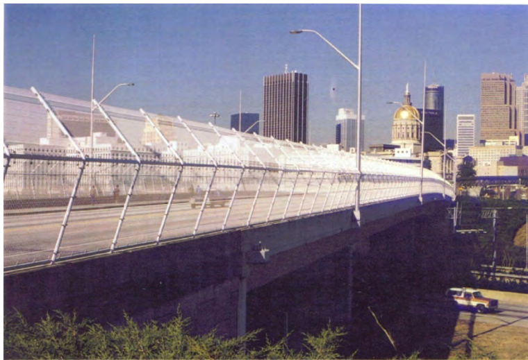
Figure 3.2 Angled Missile-proof Fencing in Atlanta, GA (photos courtesy Omega Co.)
